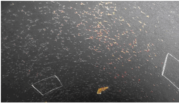
Figure 1: Distribution of internal pipe lining cracking over the crown of the pipe
