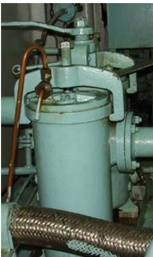
Figure 4. Lube oil suction strainers for the Main Engine Lube oil system
